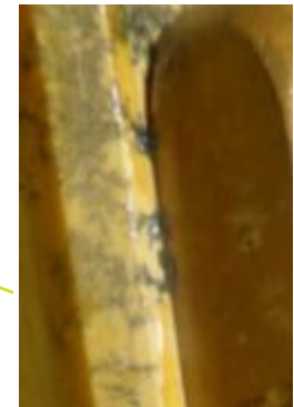
Corrosion on support structure
